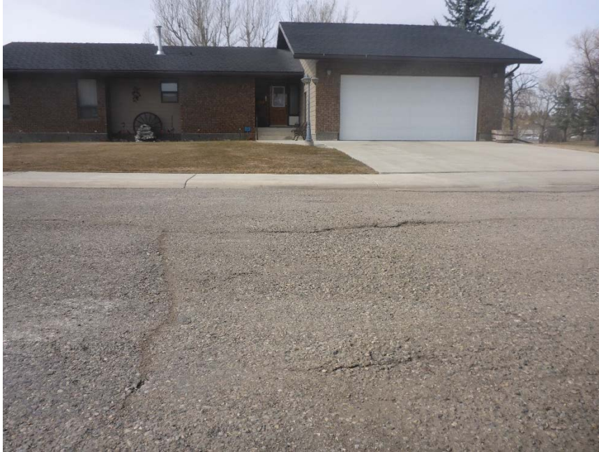
1 ST E – (2) = Station 0+012 Asphalt - Settlement
