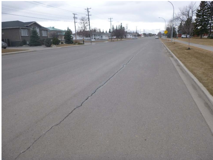
4 AVE W = Station 0+601 - 0+703 Asphalt - Longitudinal Cracking
