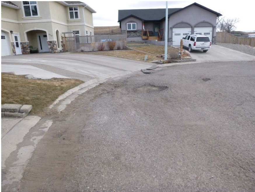
2 ST W – (3) = Station 1+500 Asphalt - Pothole
