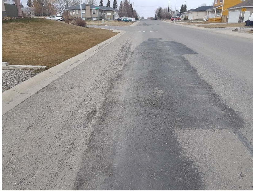
5 ST W = Station 0+180 Asphalt – Poor Repair
