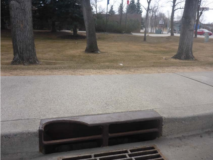
5 AVE E = Station 0+121 Damaged Catch Basin
