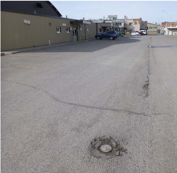
MAIN A ST W = Station 0+075 Settled Valve
