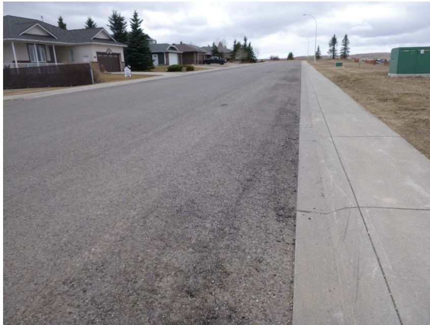
5A AVE E = Station 0+055 – 0+163 Asphalt – Deterioration
