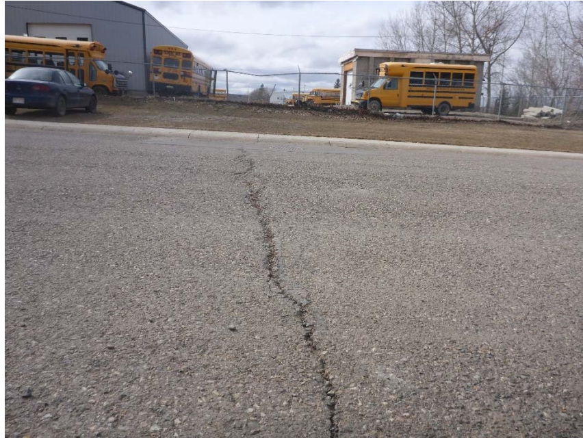
1 ST E - (3) = Station 0+185 Asphalt - Transverse Cracking
