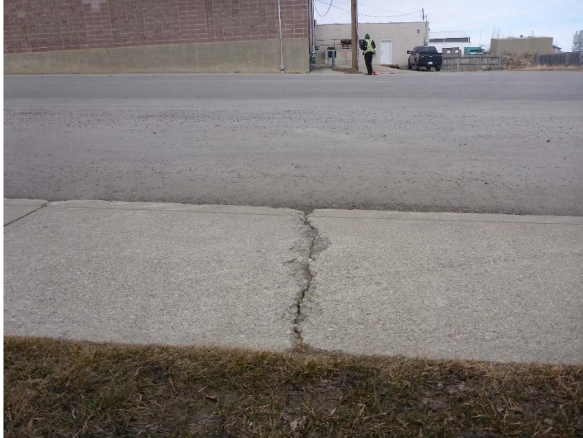
4 AVE E – (3) = Station 0+027 Concrete – Transverse Cracking
