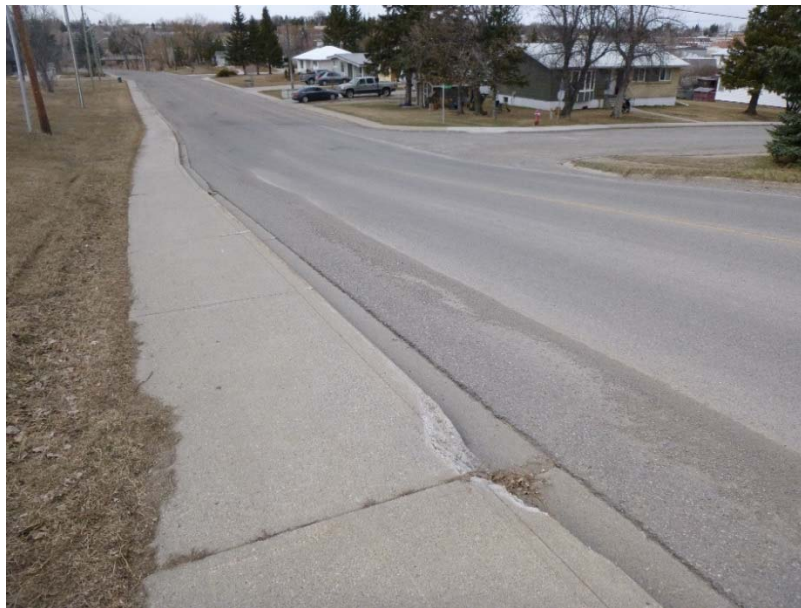
5 AVE E = Station – 0+771 Curb/Gutter – Deterioration
