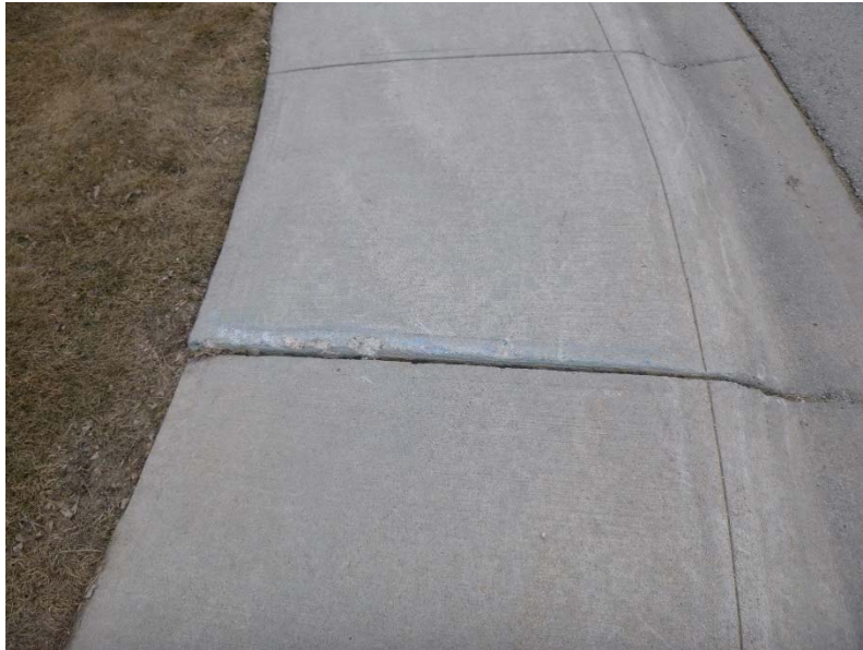
WEST CREEK DRIVE = Station 0+035 Concrete - Settlement
