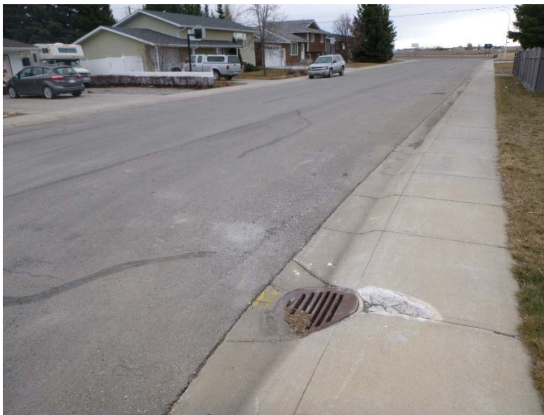
5 ST E - (2) = Station 0+003 Concrete - Spalling
