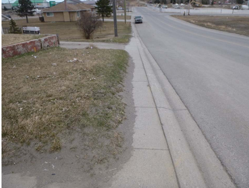
2 AVE E - (2) = Station 0+081 - 0+181 Ground Encroachment
