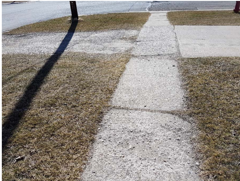
4 ST W = Station 0+229 -0+279 Concrete – Deterioration
