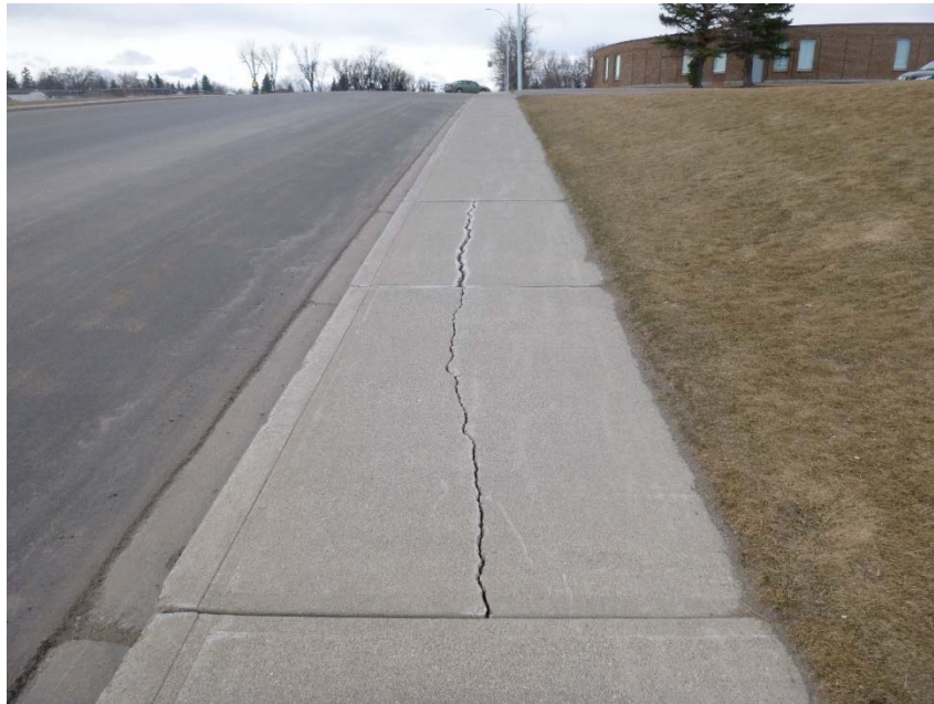
4 AVE W – Station 0+090 – 0+099 Concrete – Longitudinal Cracking
